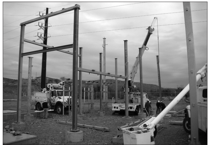
A Graham County Electric Cooperative line crew works on the Talley Substation.
