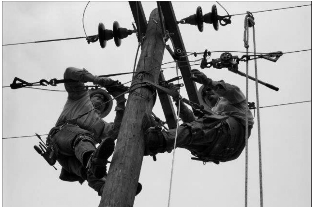
Myles Ray, left, works with Ryan Botkins on top of a power pole. Below, Myles heads out on a job.
