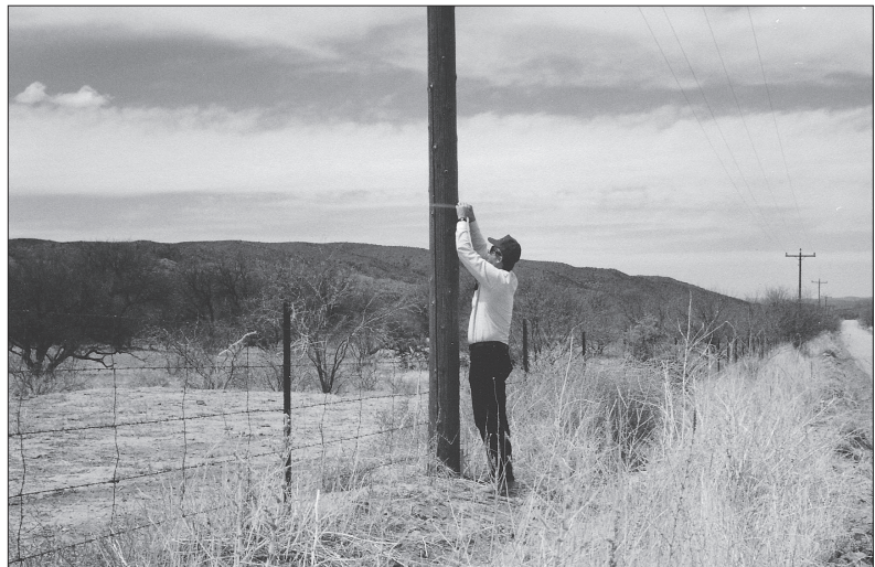
Steve marks a power pole with a red ribbon to signify that it needs repair.
