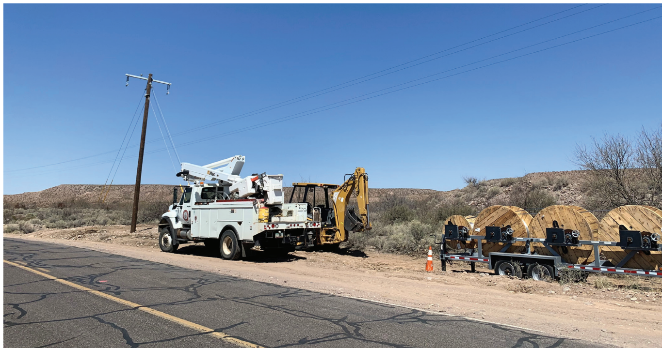
Graham County Electric Cooperative crews ready new cable for the Hillcrest to Sanchez line scheduled to be completed next year.
