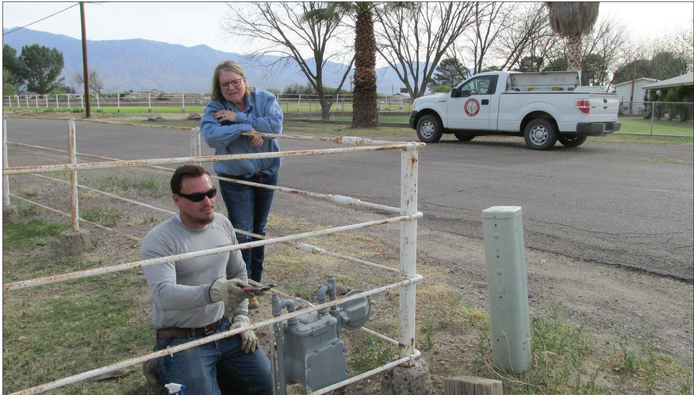
Office Communications Manager Diane Junion watches as Member Service Technician Curtis Whittle checks the pressure on a gas meter.
