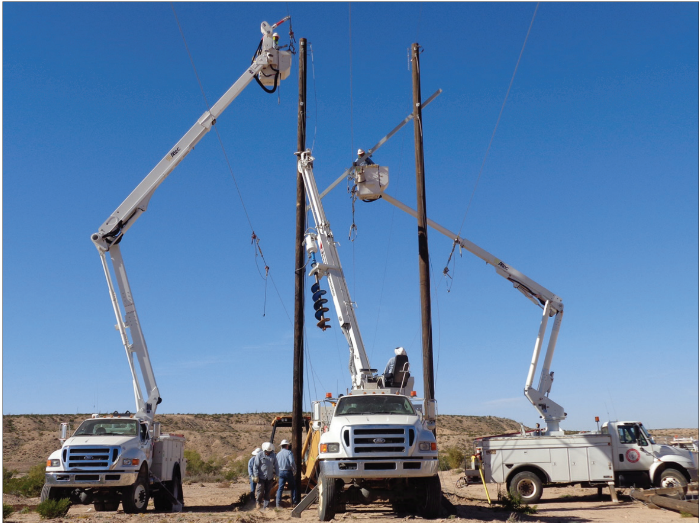
Graham County Electric Cooperative crews change out poles after inspections determine which poles need to be replaced.
