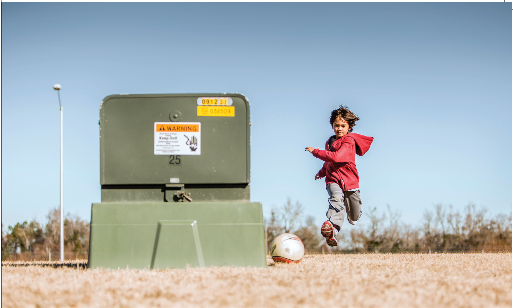
Warn youngsters not to play around or climb on the green transformer boxes that house underground electrical facilities.
